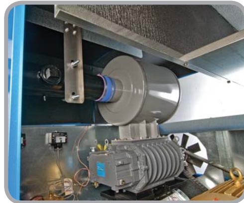
View with rear panels removed
